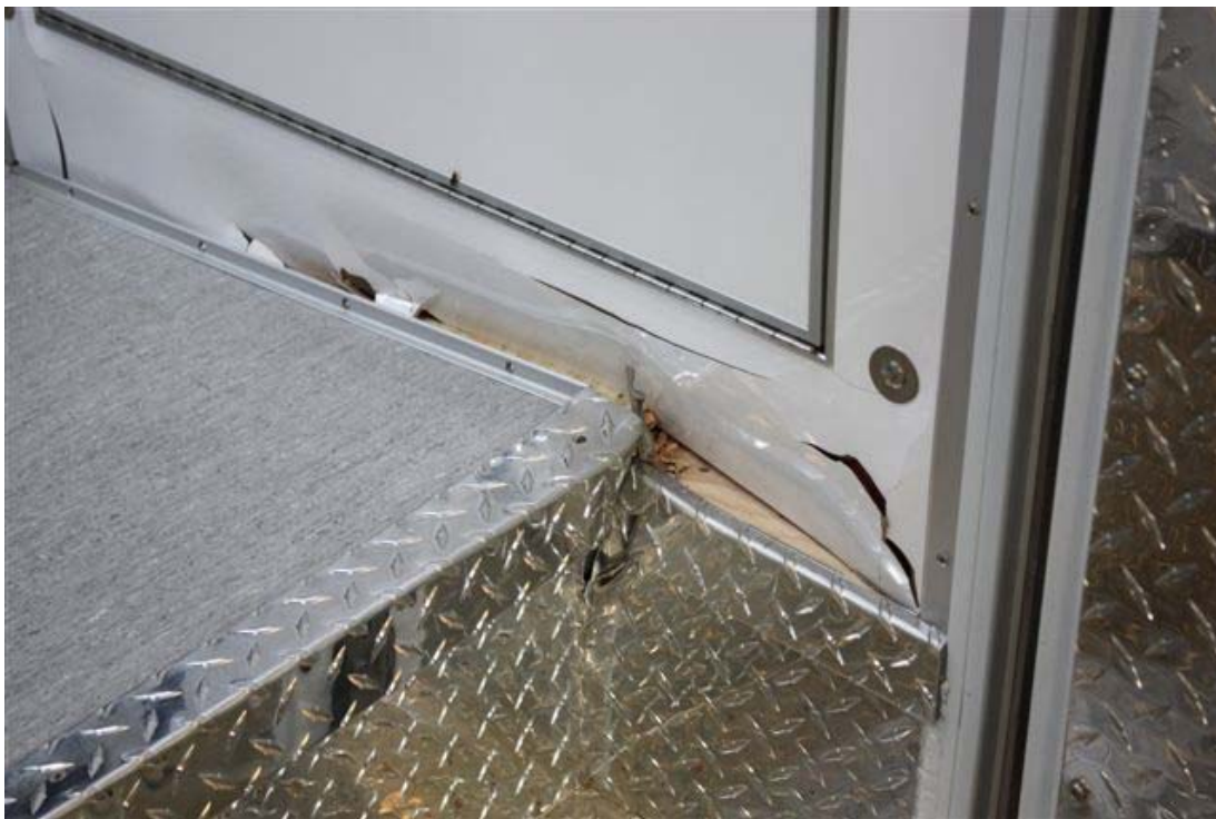
VIEW SHOWING DAMAGE INSIDE PERSONNEL DOOR (TEST 052)
